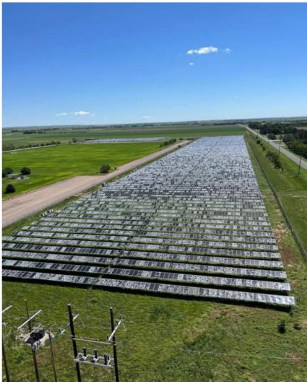
5 Megawatt solar plant destroyed by hail (solarni paneli uništeni od padanja tuče)
